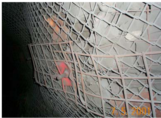
Fig. 15. Rockburst support system comprising strong meshes, mesh straps, and energy-absorbing yield rockbolts in a Canadian deep mine (photo by B. Simser).
