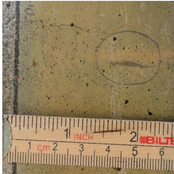
Figure 22: Example of a partly closed crack mouth (marked with grey circle) next to an open crack on the surface of Beam E. Location: 80 cm
