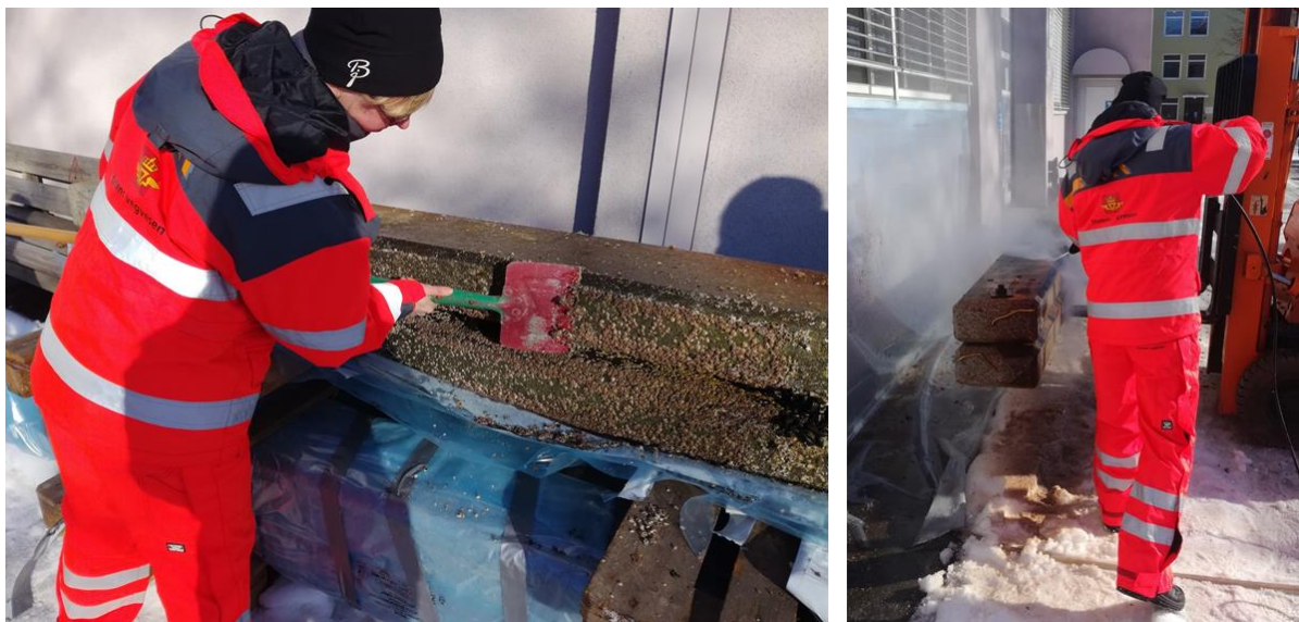
Figure 11: Surface cleaning of concrete beams. Left: Scratching of shells and algae; Right: Washing with pressure washer (15 th March 2018 – Photo: Ragnhild Moastuen)
