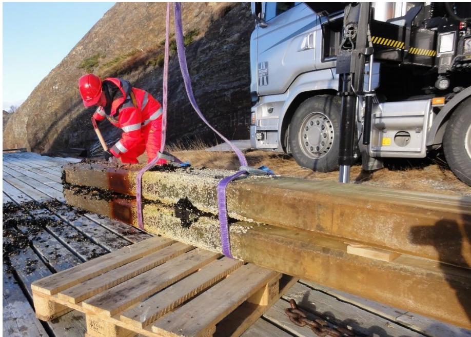
Figure 5: Removal of a pair of concrete beams and preliminary surface cleaning (14 th March.2018 – Photo: Tobias Danner)
