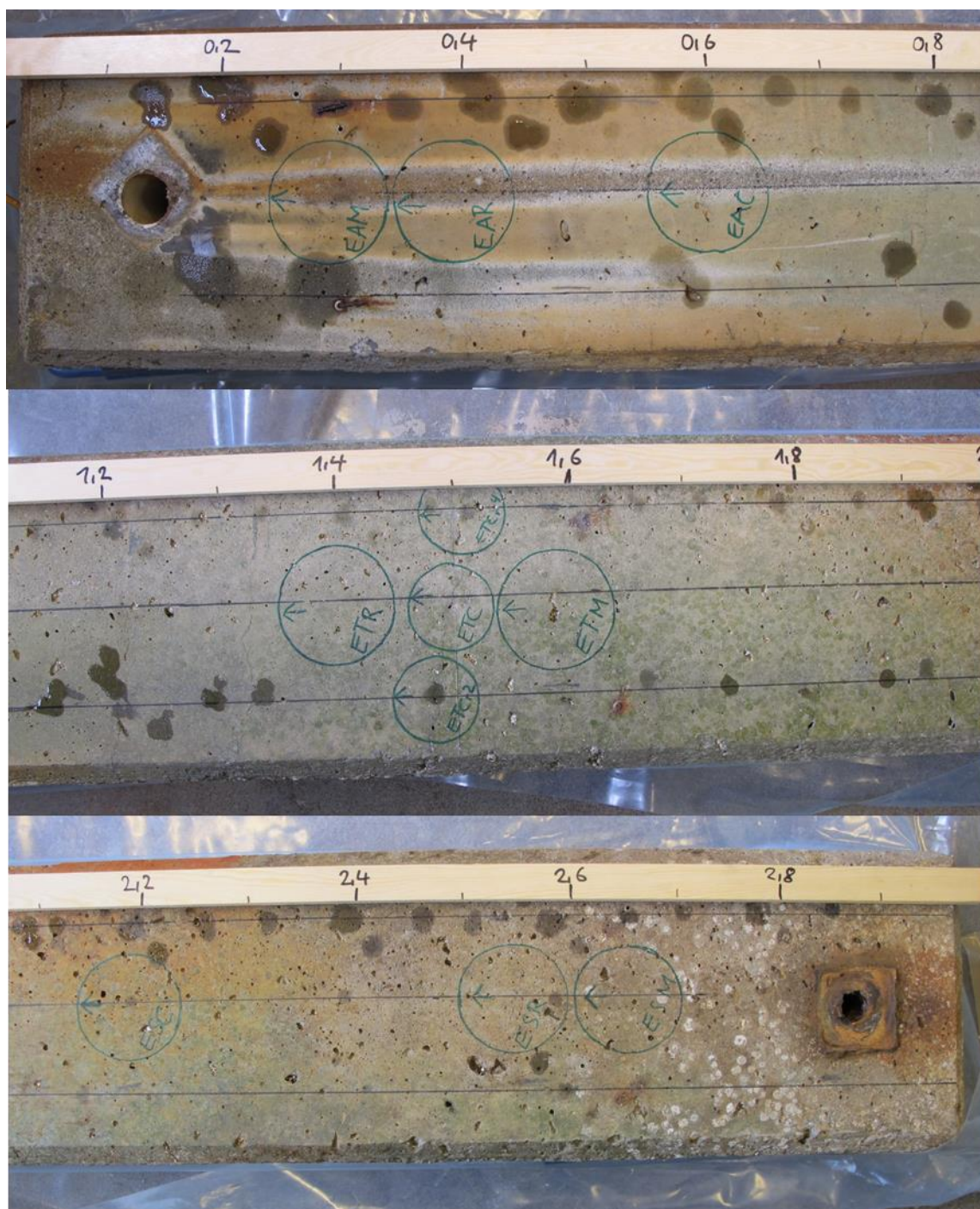
Figure 3: Location of concrete cores taken from Beam E, distance in meters (Photos: Eva Rodum)
