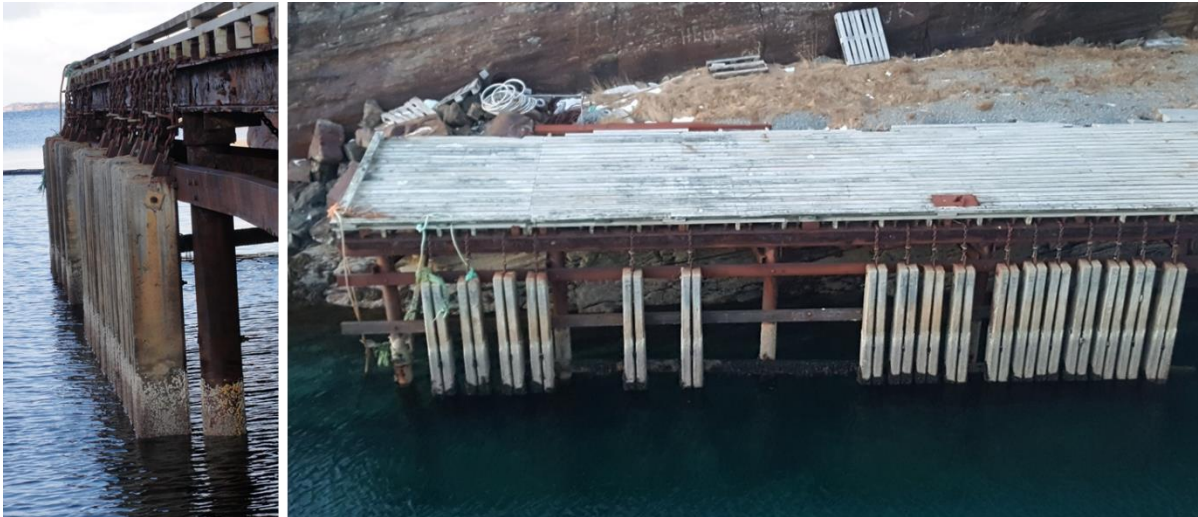
Figure 3: Field Station Sandnessjøen showing the concrete beams exposed to tidal water (14 th March 2018 – Photo: Tobias Danner)
