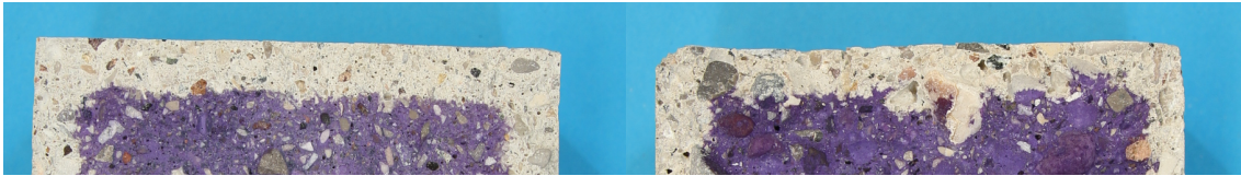
Figure 24 Left: carbonation front in mortar sample. Right: carbonation front in concrete sample.
