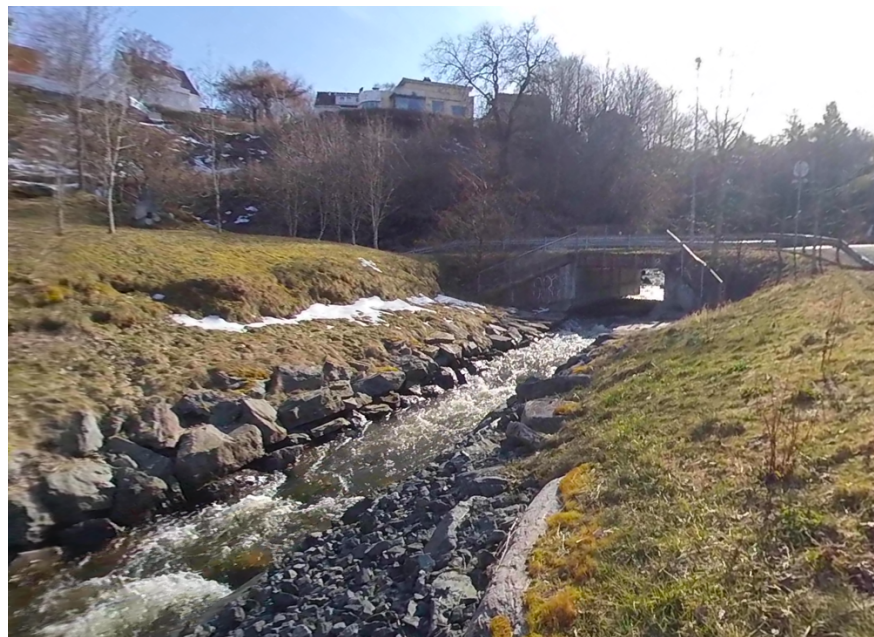
Figure 5.27 A concrete channel was built to prevent over infiltration of water (Source: Author, developed from OF, walking interview)
