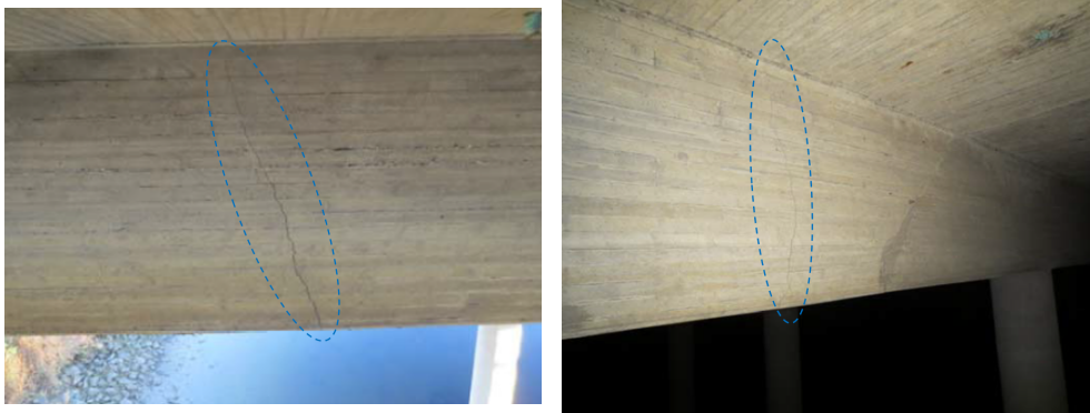
Figure 3.11: Cracks in points of zero bending moment [16]
