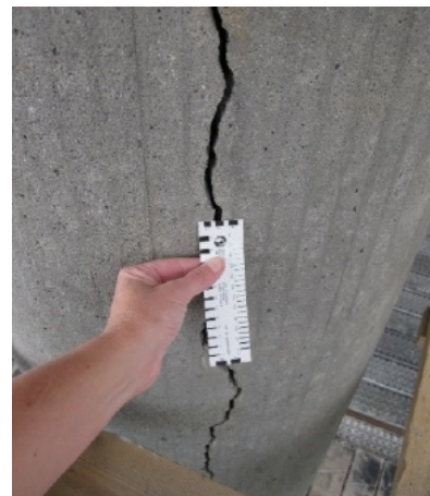
Figure 3.7: 7 mm crack width in column 3A [18]
