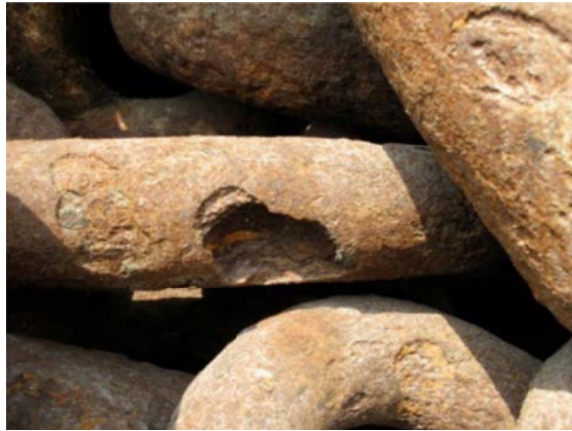
Figure 1.2: Pitting corrosion on mooring chain[8]
