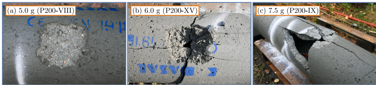
Fig. 8. Damage to P200 pipes after testing with cubic C-4 charges from position (ii), for (a) 5.0 g, (b) 6.0 g, and (c) 7.5 g.
