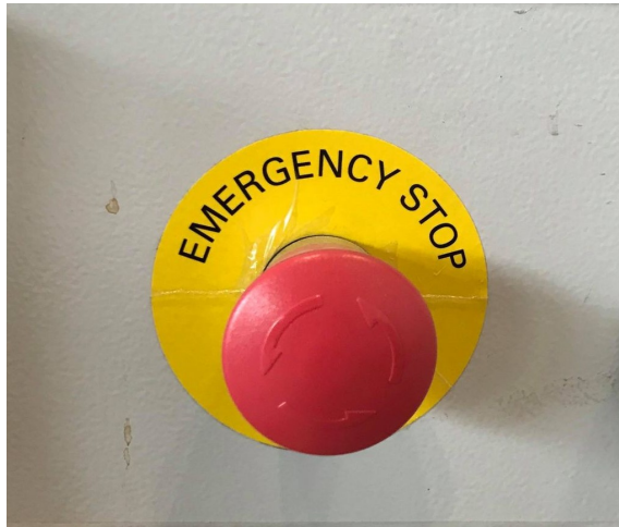
Figure 24: Emergency stop button on the automation cabinet.
