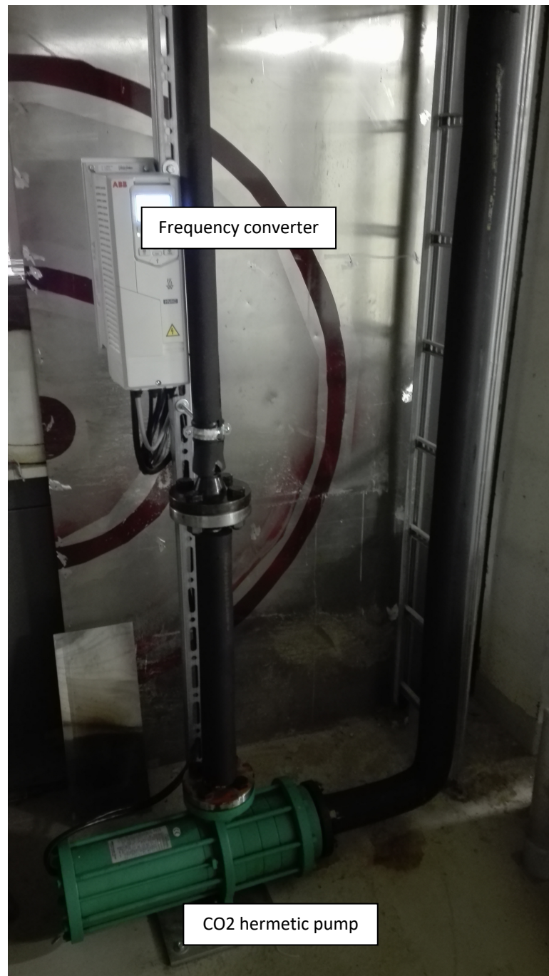
Figure 8: CO2 hermetic pump in basement
