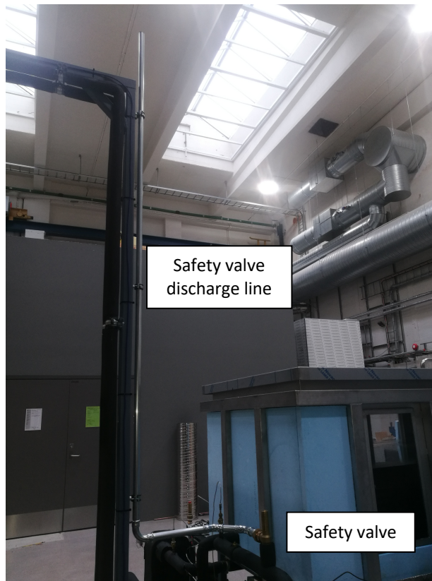
Figure 6: Discharge line from refrigerant safety valve
