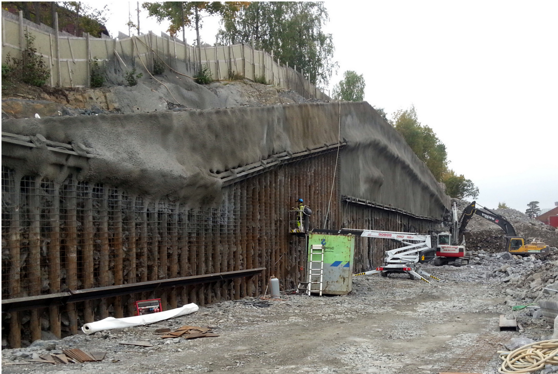
Figure 3.4.2: Bored pile wall at Avløs station. There are a total of three girders with rock anchors at different levels, from Geovita AS
