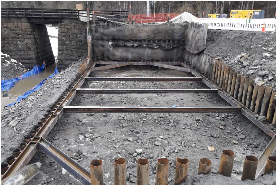
Figure 4.2.1: Construction pit for a railway foundation at Dokknes. The pipes were drilled through a railway embankment and finished in hard clay, from Geovita AS.
