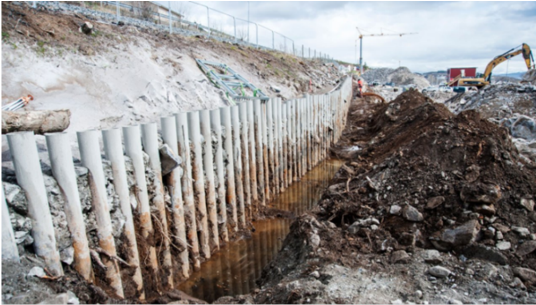
Figure 3.3.4: Steel pipe retaining system against the railway situated on the left side. On the other side, it is excavated and ready for bracing with steel beams and reinforced concrete
