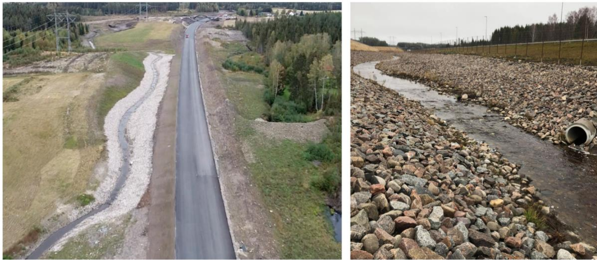
Figure 3.2 The rearranged part of Stabekken, parts of the new road and the swale on the right side of the road during the construction period (left picture, Photo: Skanska). The rearranged part of Stabekken including the culvert outlet (right picture, Photo by: Mari Gilje Lillegraven, 9 th of November).
