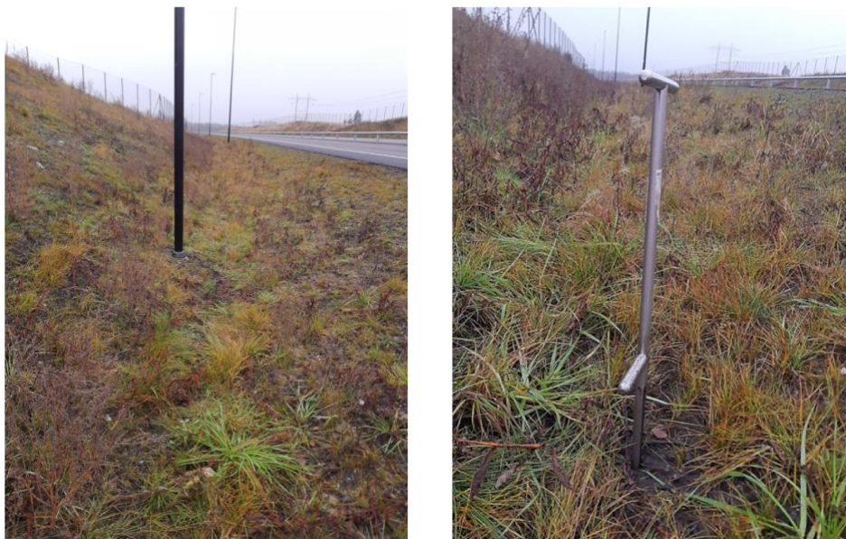
Figure 3.1 Pictures of the swale surface and its vegetation (Photo by: Kristine Bergseng, 9 th of November).
