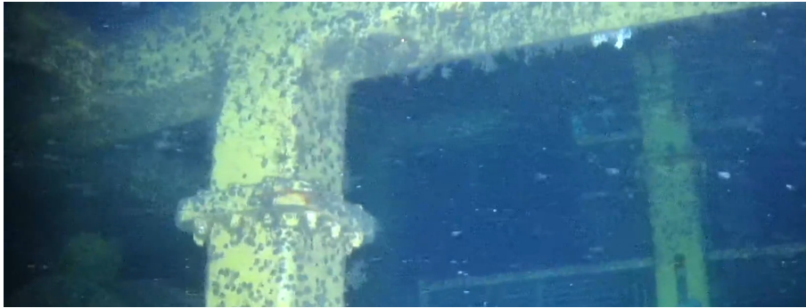
Figure 6.6: Marine growth present on a subsea structure. Footage from NTNU's EELY500 robot [11, 35, 36].
