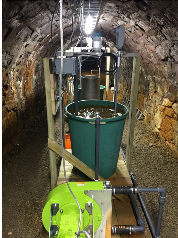
Figure A.1 Trondheim municipality’s system in 2018 and the beginning of January 2020. The lime green pump is taking water in from the tunnel and into the first tub. It passes on further through lime in the metal cylinder in the middle, before it goes into the final open tub and finally exits back into the tunnel.
