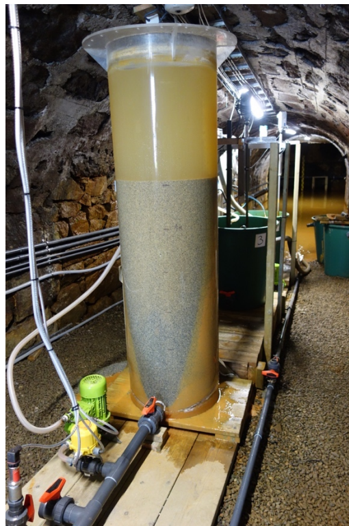
Figure A.3 Trondheim municipality's system that was installed sometime between March 22 nd and May 24 th 2019, with a plexiglass pipe filled with lime.
