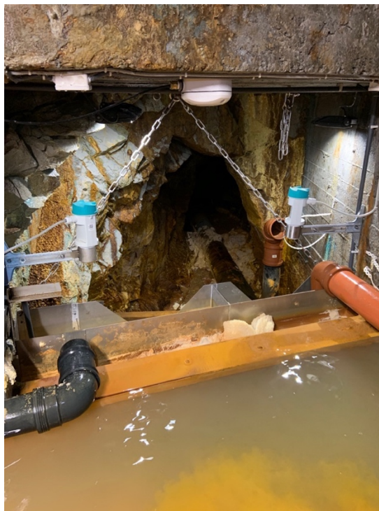
Figure A.10 The threshold where water from inside the tunnel runs over the edge when the water levels are high enough. This is also where the water from the sampling points “first collection” and “second collection” are led. Samples here were taken just over the threshold.
