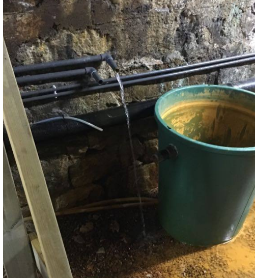
Figure A.11 The hose bringing untreated tunnel water in from inside the tunnel. This was the sampling point of the tunnel water when there was no sampling possibility in Trondheim municipality's systems due to closed pipes.
