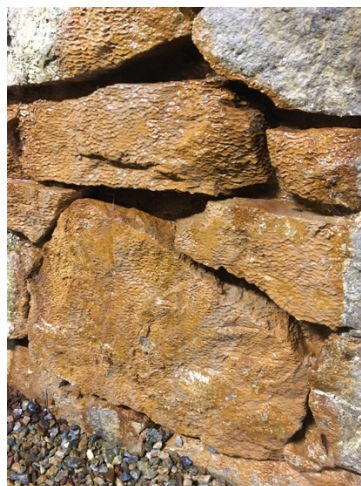
Figure A.5 Water coming through the tunnel wall. This is the sampling point "tunnel wall", and samples were taken of a weak stream approximately in the middle of this picture, not visible due to the shadow. The sampling point "left tunnel wall" was not photographed, but was similar to this.
