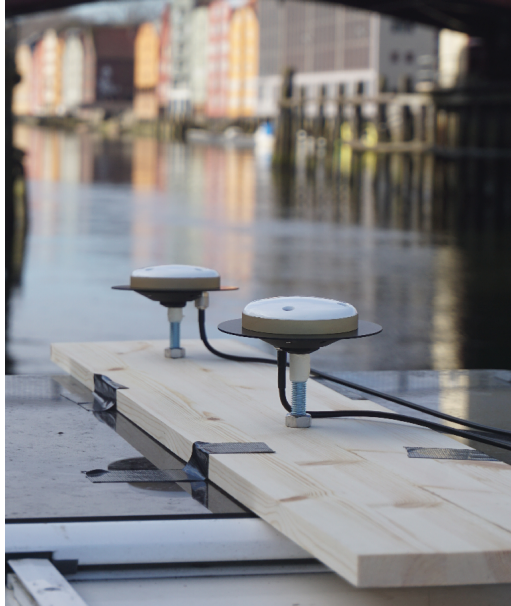
(a) Dual antennas mounted on the roof of Havfruen
