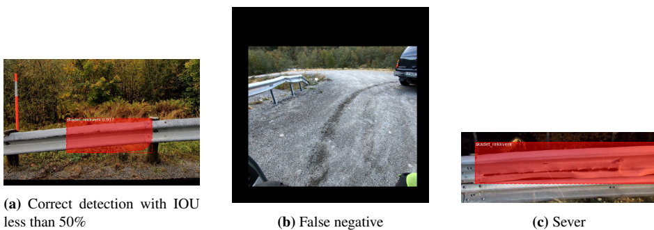
Figure 6.2: Severe damage to the railing
