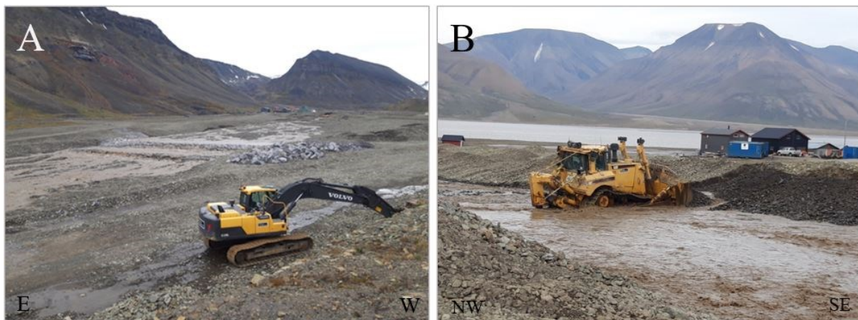
Figure 37: Immediate maintenance had to be done during floods. A) After the first minor flooding on June 24 th , an excavator was used to reassemble damaged sills. B) July 27 th , discharge 6.2\text{m}^3/\text{s} . Bulldozer performing critical maintenance downstream Veg 600 to keep the river from eroding the levees and threatening to flood the red pump-house.
