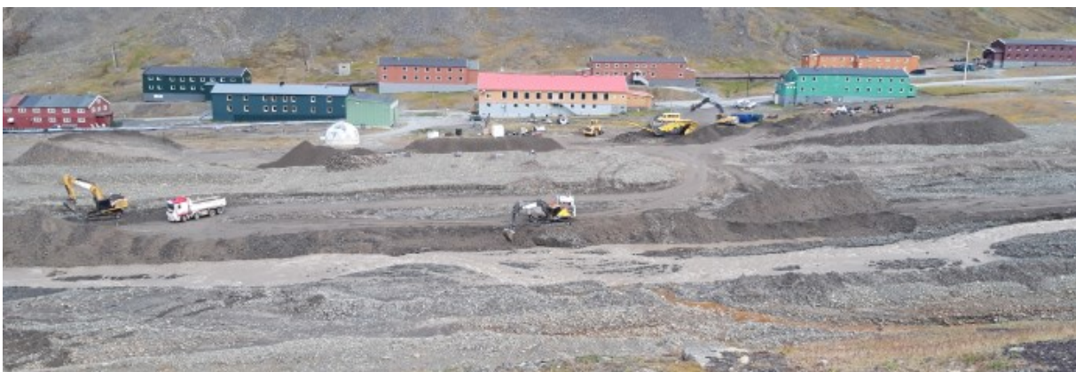
Figure 36: Excavation of fluvial sediments next to Nybyen, deepening the channel to keep the river from migrating. The material is intended to be used in the construction of landslide mitigation in Lia. Picture from August 10 th .
