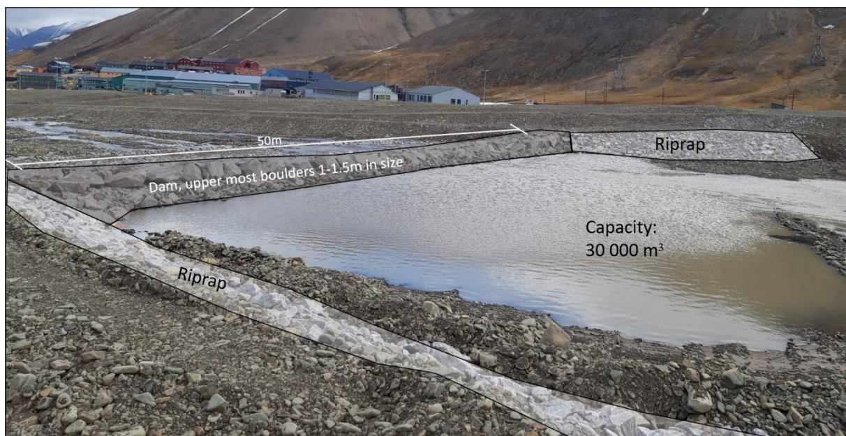
Figure 14: Annotated picture of the Sedimentation dam, riprap on both flanks to avoid undercutting. The dam consists of large boulders of blasted granitic gneiss, with an apron of smaller boulders downstream. The large boulders allow water to percolate through, while reducing the energy and allow bedload to settle.
