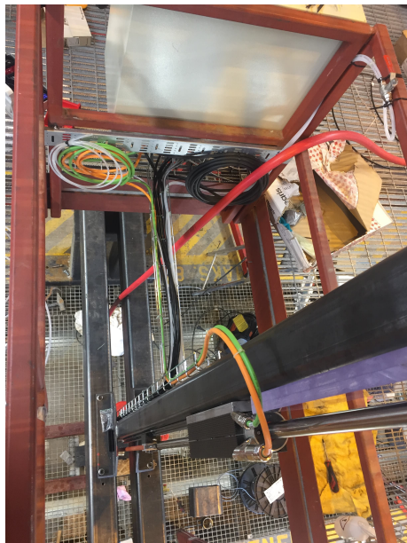
Figure B.21: Motor and sensory cables attached to the cable canal running into the junction box.
