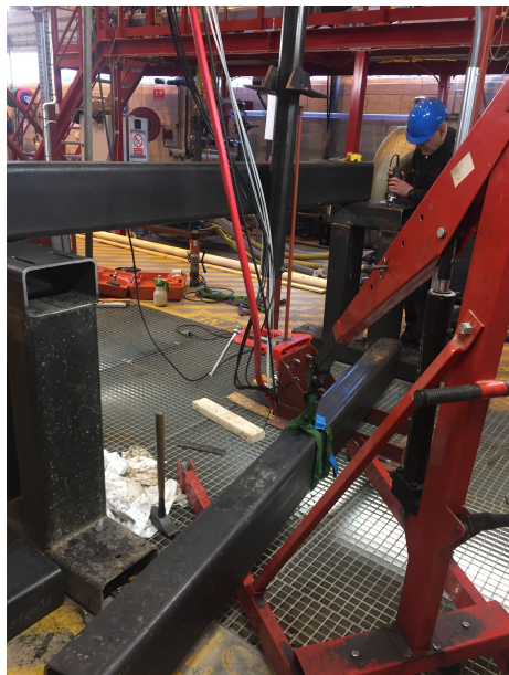
Figure B.13: Mounting of supporting structure for counterweight and motor assembly. Making grooves in the bottom foundation in order to have adjustment possibilities of the structure. Completed in order to properly center the linear motor above the drillstring.
