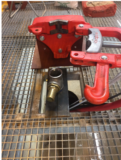
Figure B.5: Surface slips and casingstring mounted to steel garters at surface
