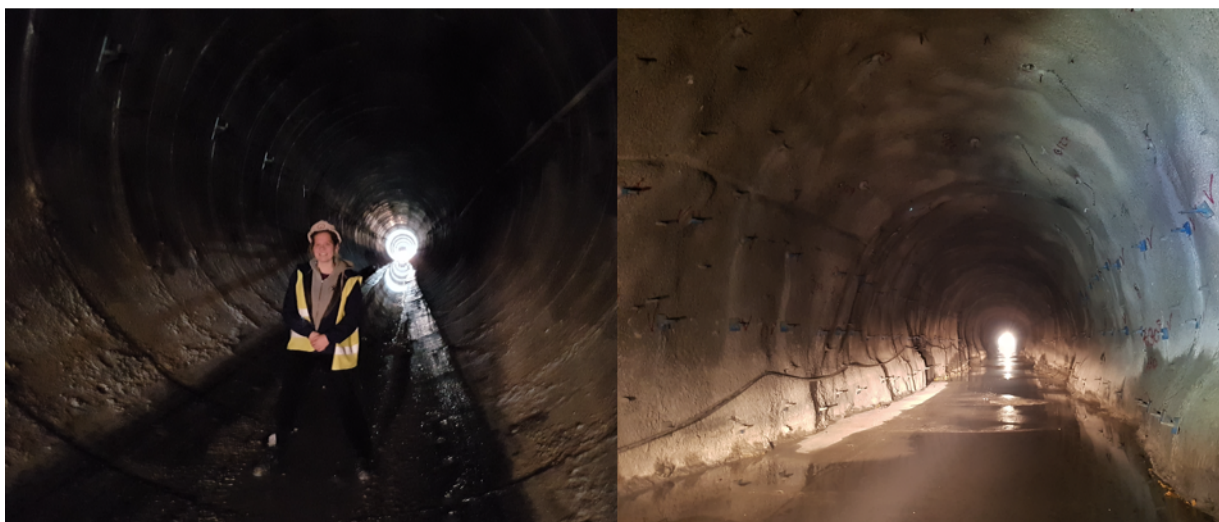
Figure 4.5. Tunnel profiles along the headrace tunnel. The left photo is from the part excavated by TBM, while the right is from the drill and blast section (Photo: Runa B.Freng 27.03.2019).
