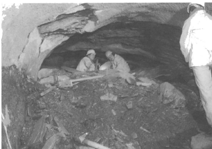
Figure 2.3. Debris from fallout and slides in the Chingaza tunnel. Note the broken shotcrete lining (Brattli and Broch, 1995).
