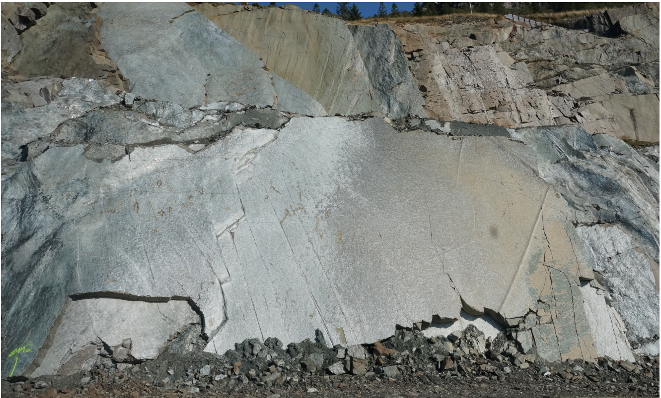
Figure 4.17: Photo of the plane failure used to calibrate the joint strength parameters of a serpentinized surface. The bench is about 15m high.
