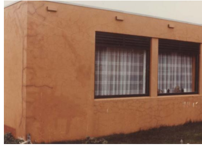
(b) Characteristic map cracking for ASR (Guðmundsson, 2007).
