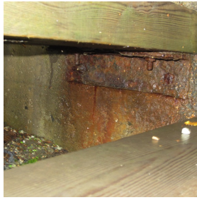
(b) Smudged Corrosion.
