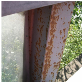
(h) Scattered Corrosion and Undefined Number of Instances.
