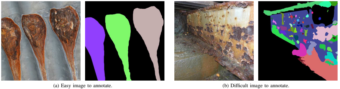
Fig. 2: Instance segmentation masks for two images. (a) Three instances are immediately recognized, and their boundaries are sharp, making it easy to annotate the image. (b) With a large number of potential instances, some areas more severely corroded than others, boundaries being smooth, etc., this is a very challenging image to annotate. Black indicate no corrosion, i.e. background. Instances are assigned random colors and have no further interpretation.
