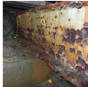
(i) Heavy Corrosion Surrounded by Light Corrosion.
