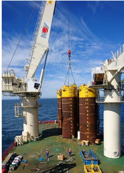
Figure 3.27: Installation of suction anchors at Hywind Scotland, done by TechnipFMC with the DSV "Deep Explorer" (FFU, 2018)
