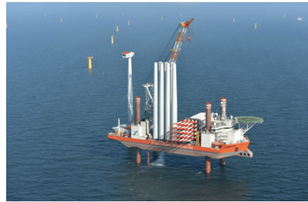
(b) Fred. Olsen Windcarrier's "Bold Tern" installing a wind turbine at the Butendiek wind farm in the German North Sea (Fred. Olsen Windcarrier, 2015)
