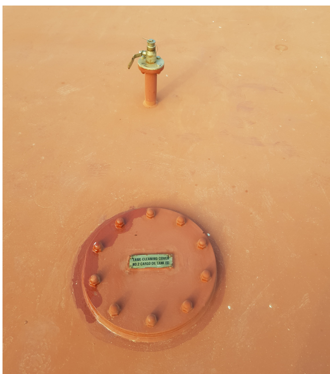
(b) Picture of vapour control valve for C.O.T 2(S)
