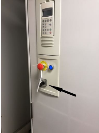
1e - Pump frequency drive and power switch
