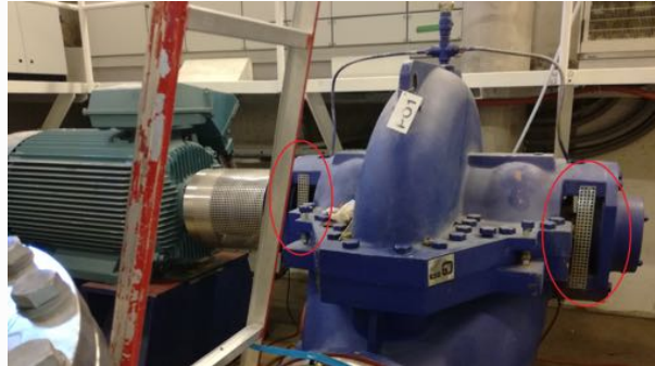
1m - Pump seal
