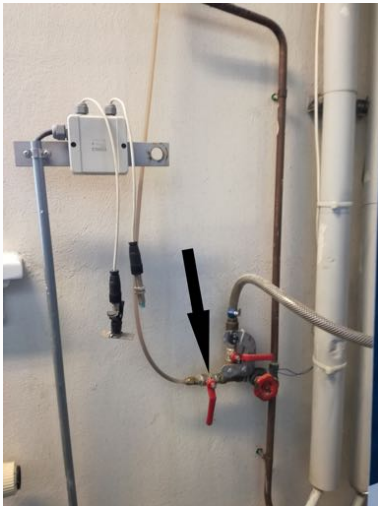
1k - Water tap to prime the differential pressure transducer
