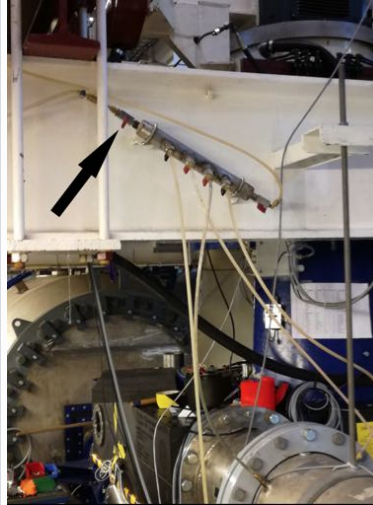
1j - Inlet pipe pressure manifold
