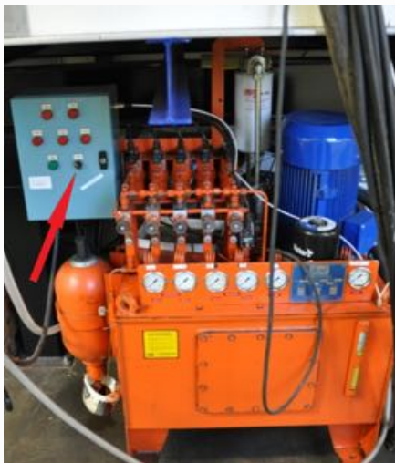
1c - Hydraulic pump unit and pressure dials
