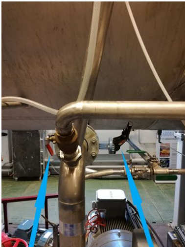
1g - Draft tube tank bleed- and drain valves
