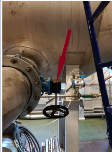
1f - Draft tube tank pump outlet valve
