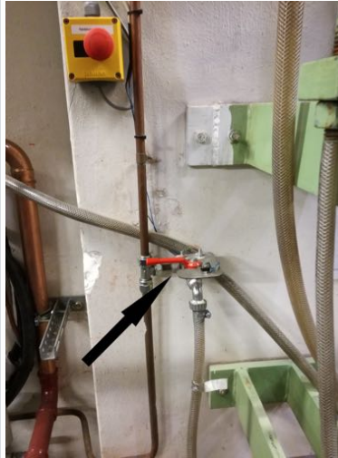
1b - Water tap for the hydraulic system cooling water
