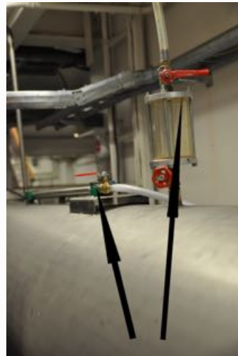
1h - Inlet (and outlet) pipe bleed valve
