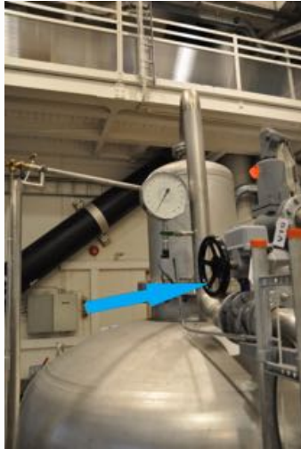
1a - Bleed valve on the pressure tank (V18)
