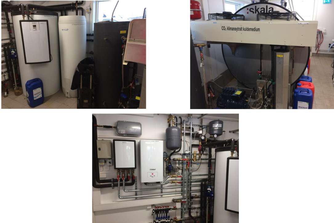
Figure 17: The electric boiler, storage tank and water heater at the milk barn. Photos: Dan Remi Antonsen.
