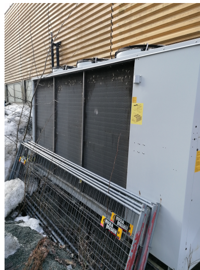
Figure B.1: AMC Chiller
