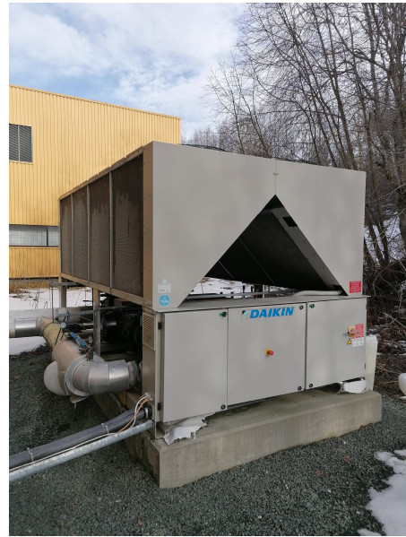
Figure 3.5: DAIKIN EWAD 480D-SL Chiller
