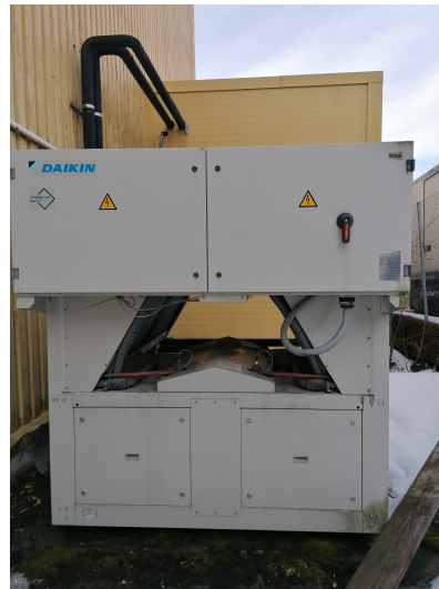
Figure B.4: DAIKIN EWYQ 150 DAYNB Chiller
