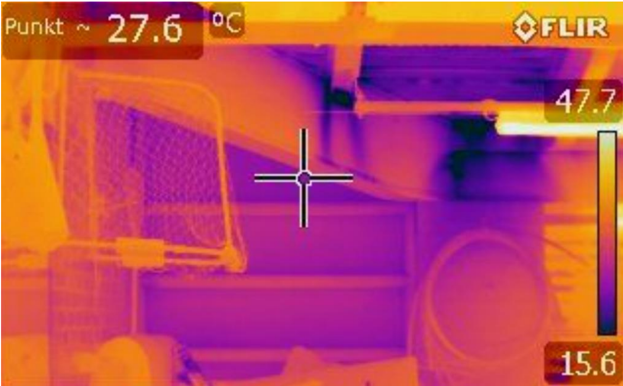
Transition between external walls and ceiling (for a dark purple color the surface temperature is 15.6°C. Photo: Ole Smedegård):
