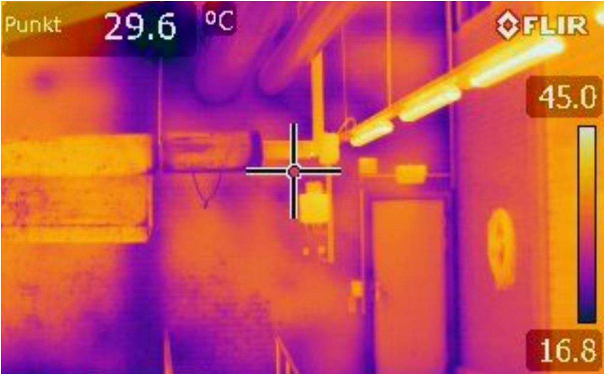
External wall showing thermal bridges at the studs (for a dark purple color the surface temperature is 16.8°C. Photo: Ole Smedegård)
