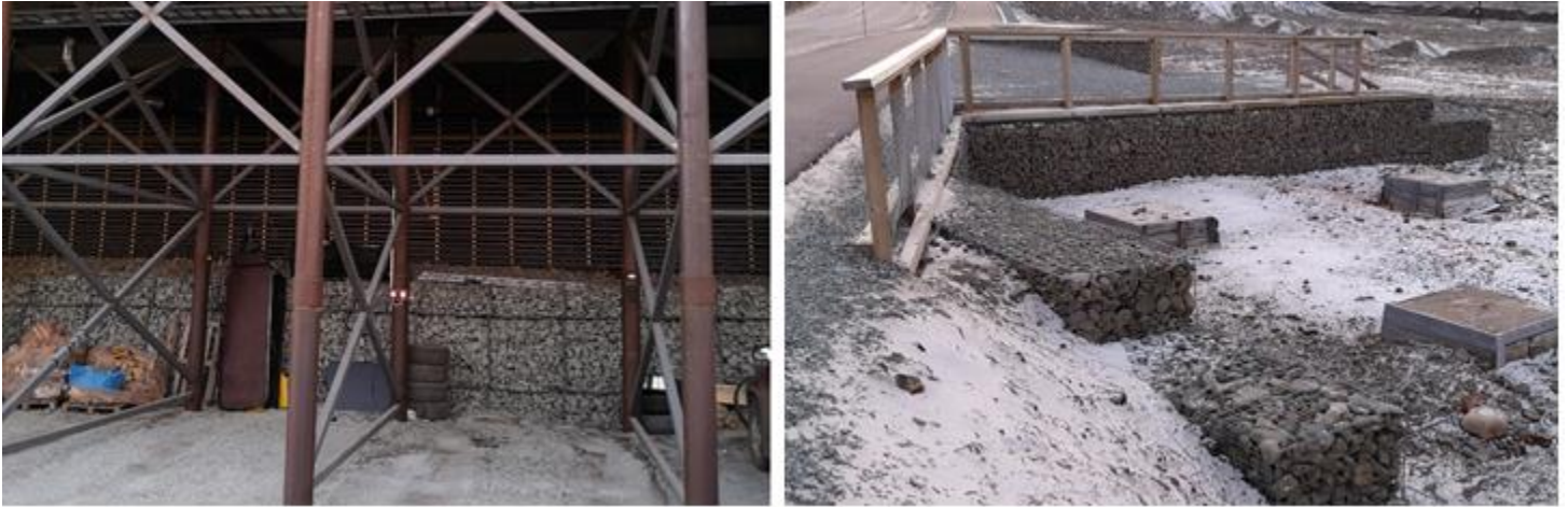
Figure 32: Use of gabions in Longyearbyen (structural with imported rocks on the left and architectural with local rocks on the right)
