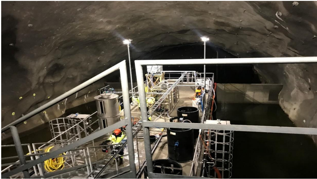
Figure 1: The sedimentation basin and pilot setup in Bjørnegårdstunnelen (BT). The second water collection was done here, in the basin on the left side
