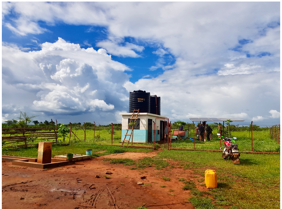
Solar-powered water pumping system in Endagaw chini village, Mbulu district
