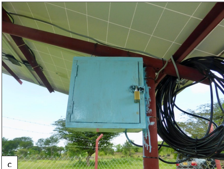
Figure 25: a) Plastic box containing gateway, cable with resistance and Neuron mA Digitizer b) System components inside wooden box, c) Wooden box attached to solar panels of pumping station
