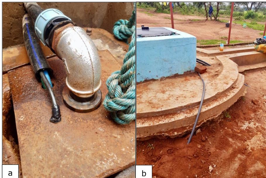
Figure 27: a) Cable of UNIK5000 entering the borehole, b) Tube containing the cable of UNIK5000
