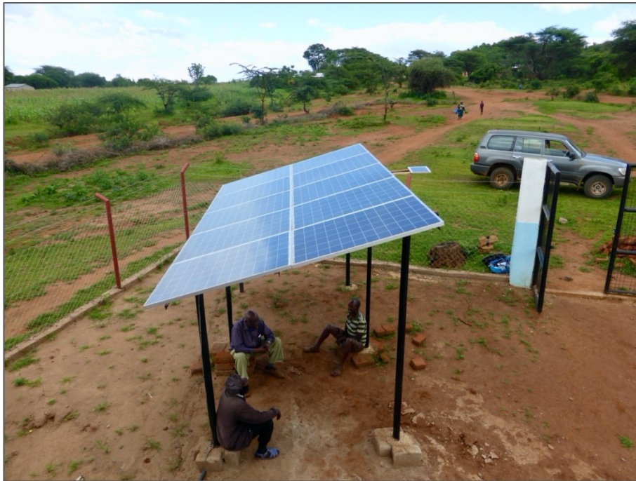
Figure 8: PV-panels at Mewadani pumping station
