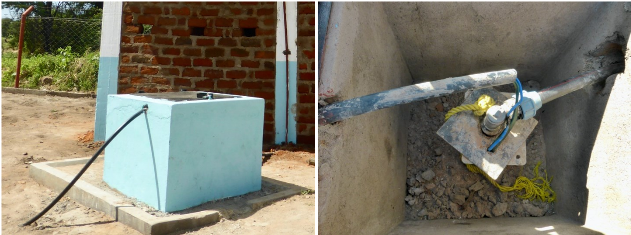
Figure 50: Wellhead at Hilamoto pumping station
