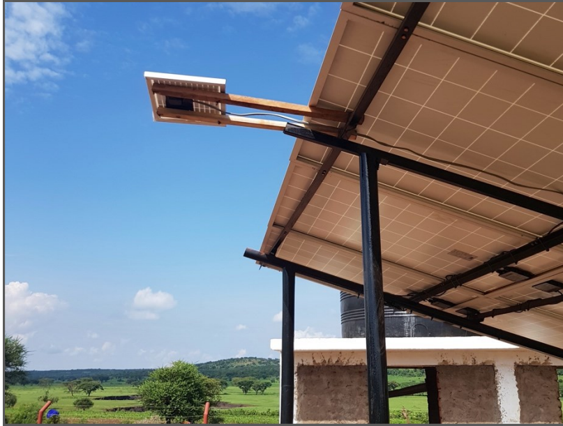
Figure 26: Solar panel of remote monitoring system attached to solar panels of water pumping station
