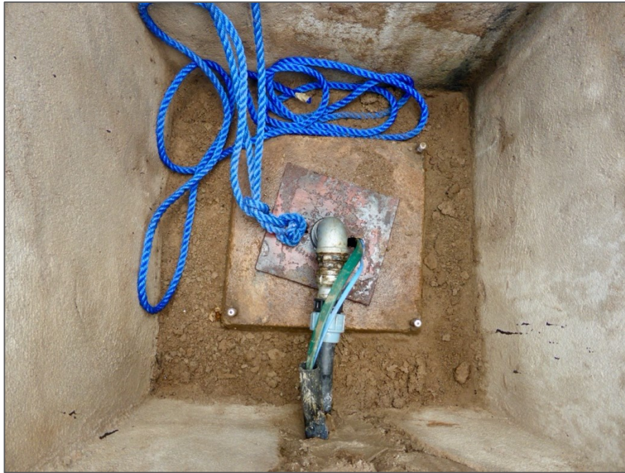
Figure 10: Top of borehole at Isene pumping station
