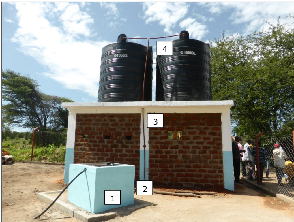
Figure 32: Borehole and water tanks at Hिलamoto pumping station. The numbers 1-4 illustrate different sections for friction loss measurements
