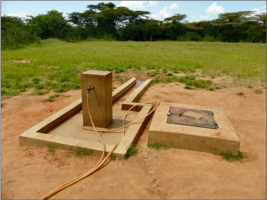
Figure 12: Water tap at Gidbyo pumping station
