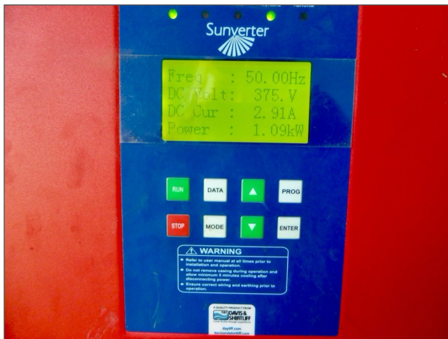
Figure 9: Dayliff Sunverter at Endanachan pumping station
