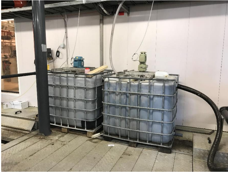
Figure 3.4 Coagulation and flocculation reactors of the pilot plant.
