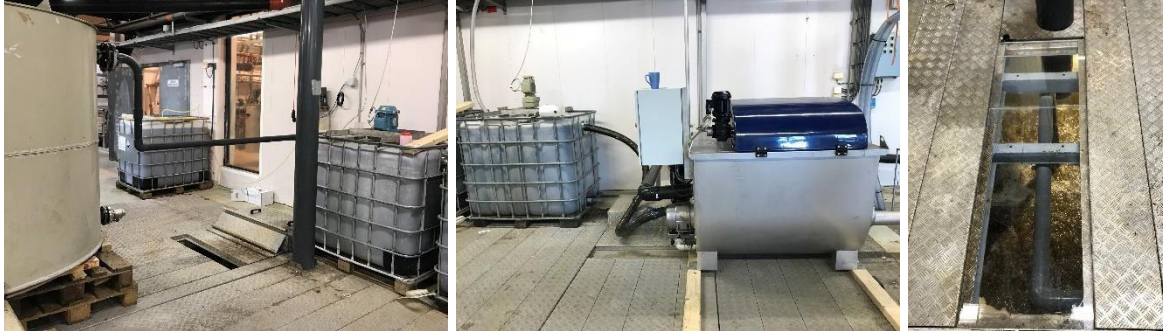
Figure 1.2-1.4 The pilot installation at FREVAR
