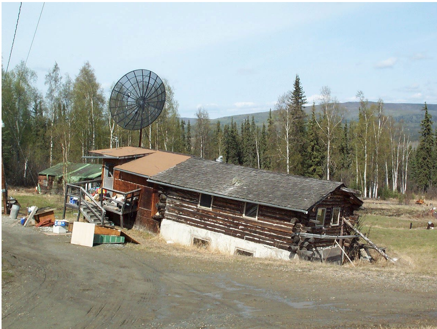
Figure 2.5: Settlements due to thawing of ice-rich permafrost in Fairbanks. Photo by Romanovsky (2018).
