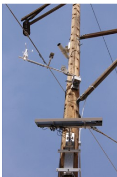
Figure 2.11: Span Sentry monitoring system from EDM [19]
