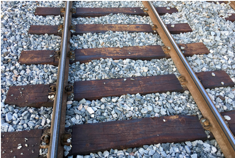
Figure 2.2: The track superstructure: Rails, sleepers (in wood), fasteners securing the rails to the sleepers, and the ballast stones. The railpads are not used in this configuration, but are more often used with concrete sleepers.
