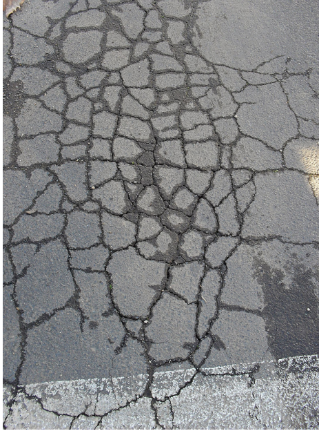
Figure 2.1: Alligator cracks containing moisture, which can be a symptom of a weakend soil underneath. "Asphalt deterioration" by Bidgee is licensed under CC BY 3.0.
