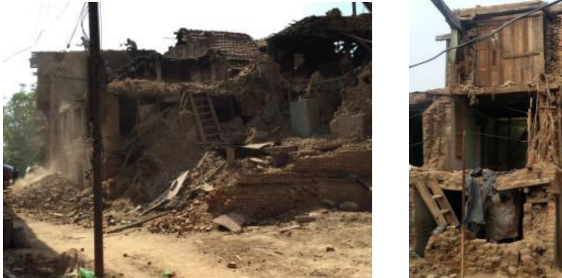
Figure 9: Damaged caused by Earthquake 2015 in Thecho (Source: Rebuilding Settlements with Communities in Thecho and Machhengoan)
