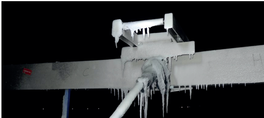
Figure 31. Photo of the ice accretion and the system after the test on the 14 th of February 2012.
