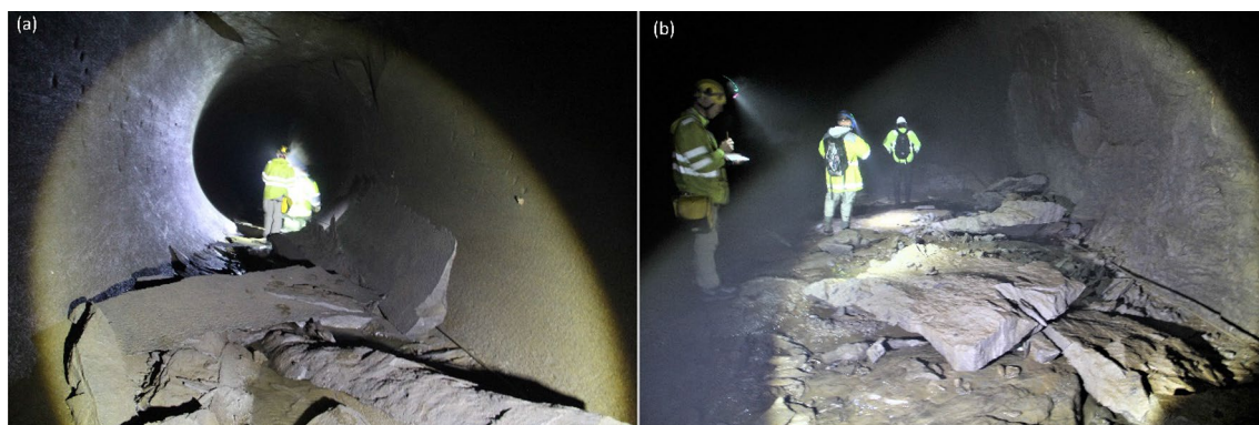
Fig. 16 Block falls registered in a hard crystalline rock (Trondhjemite) and b schistose phyllite during inspections of unlined pressure tunnel of a power plant in Norway
