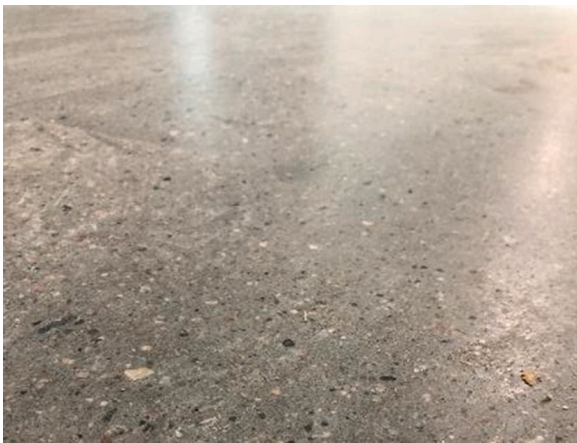
Fig. 7. Finished polished concrete in PHT, with embedded pex-pipes for low temperature heating and high temperature cooling. Image courtesy of Skanska.
