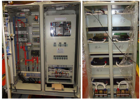
Fig. 15. Motor starter and battery panel
