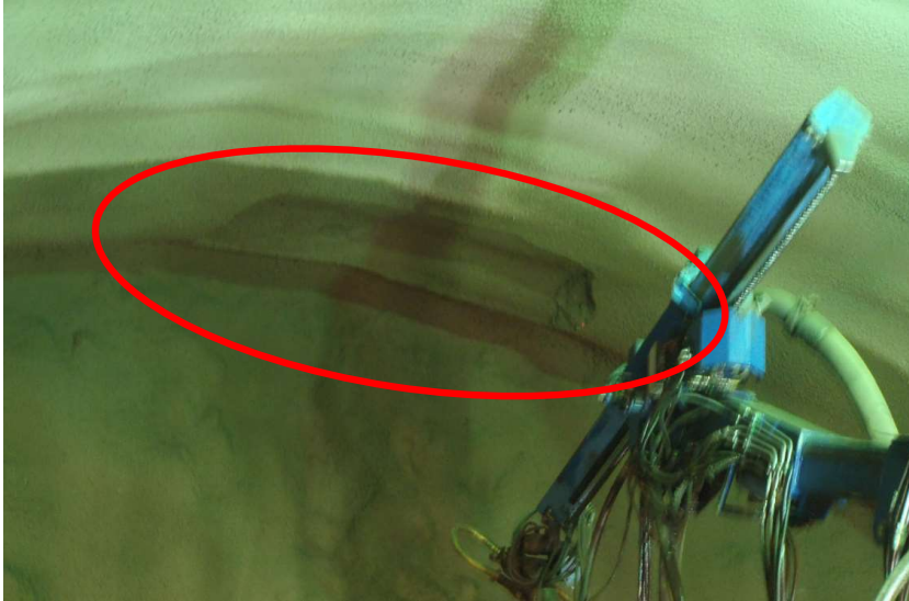
Figure 8 – Photograph showing area where sprayed concrete has fallen from tunnel crown, cause unknown but likely sprayed concrete failed under own self-weight (photograph Nicholas Trussell)
