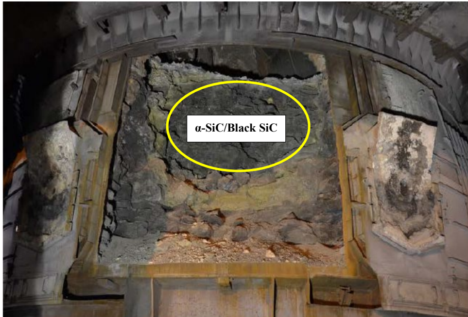
Figure 2.1.5. Status of Si furnace after opening the outer lining [15].
