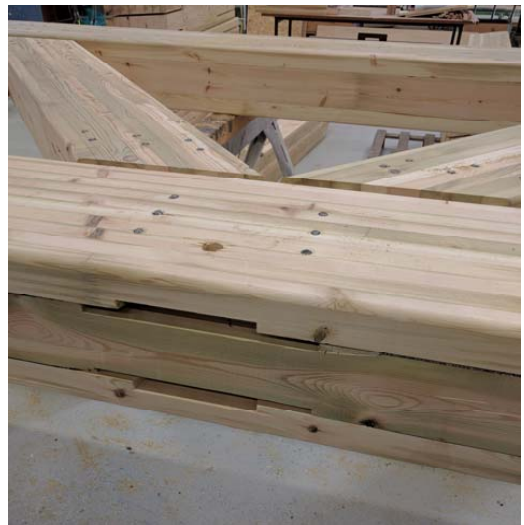
Figure 10: Physical result. The lower chord
