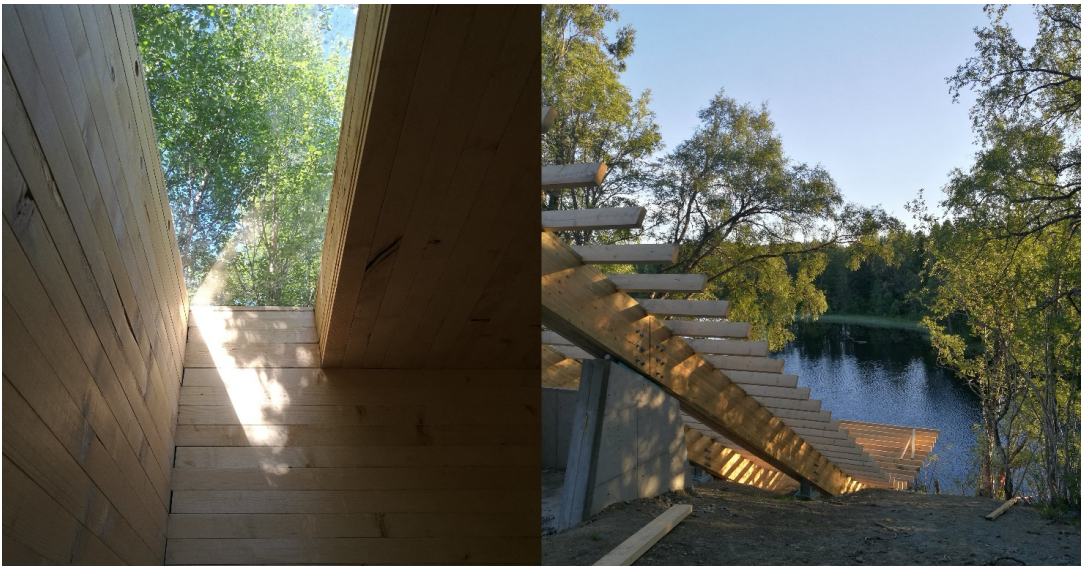
Figure 18: The sauna (mostly L-nodes) on the left side and the water ramp with secondary connection and primary extension nodes.
