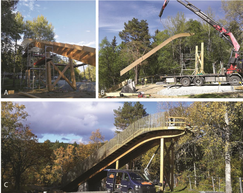
Figure 70: The top pictures show the assembly of the load-bearing structure. The platform and railing were fabricated on-site.
