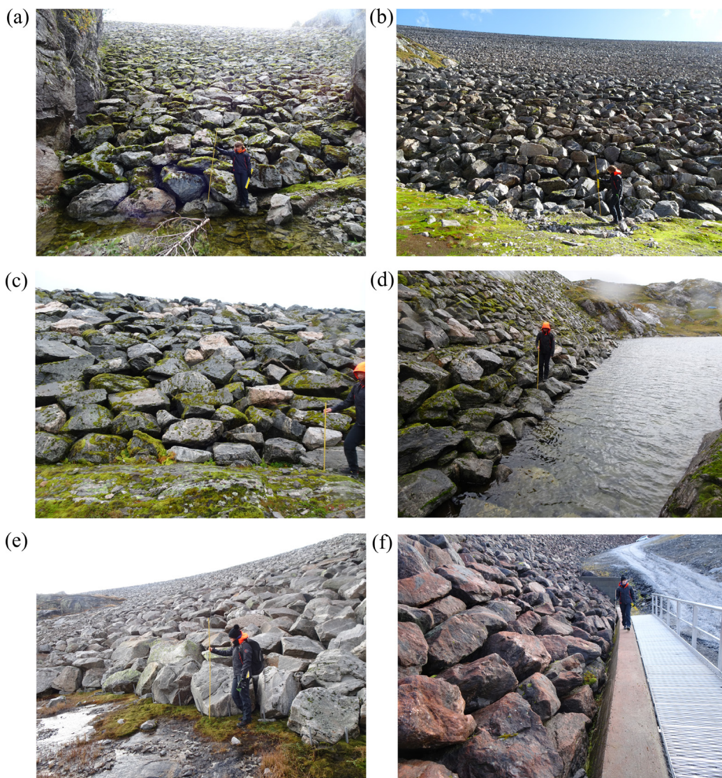
Figure 7. Depiction of existing conditions of placed riprap toe sections. Category 1 at dams (a) Fjellhaugvatn dam (b) Oddatjørn dam and (c) Skjerjevatnet main dam. Category 2 at (d) Skjerjevatnet main dam. Category 4 at (e) Storvass dam. Category 5 at (f) Akersvass dam.
