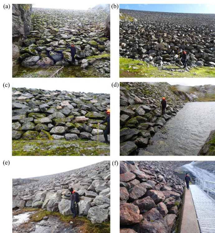
Figure 15. Depiction of existing conditions of placed riprap toe sections. Category 1 at dams (a) Fjellhaugvatn dam (b) Oddatjørn dam and (c) Skjerjevatnet main dam. Category 2 at (d) Skjerjevatnet main dam. Category 4 at (e) Storvass dam. Category 5 at (f) Akersvass dam (Adopted from Ravindra et al., 2019a).
