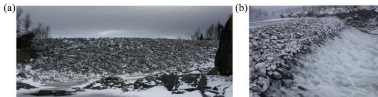
Figure 9. (a) Image of the test rockfill embankment (M1) from the test site downstream of Røssvatn, southern Norway prior to testing; (b) Image of the test dam during testing (Image courtesy: EBL Kompetanse (2006) and published in Ravindra et al., 2019b).
