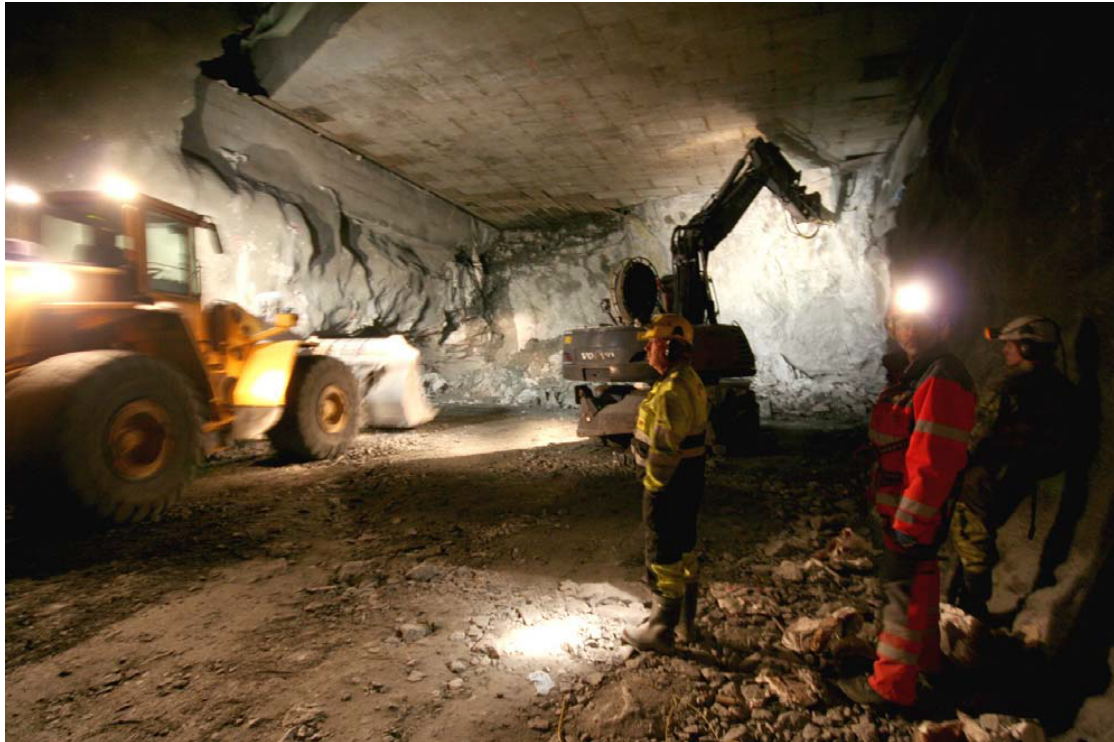
Figure 4.4: Typical construction face of drill and blast tunnelling, this picture correspond to the construction phase of Grønalia Tunnel (source: NPRA (2012))
