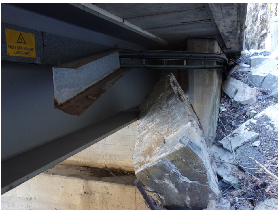
Figure 5.4: Boulder on bridge beam
