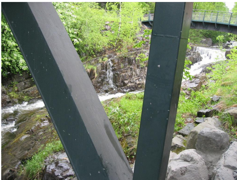
Figure 5.2: Example of the coating of a bridge assessed as fair. Pinhole application errors with zinc oxide visible over large areas can make the bridge assessed as fair
