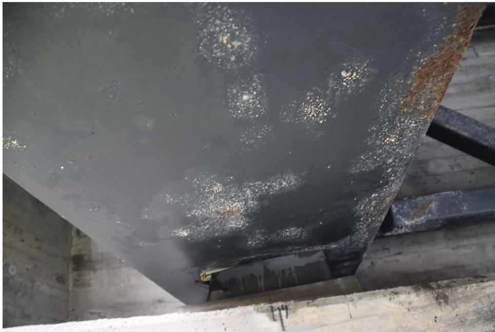
Figure 5.3: Example of the condition of a bridge assessed as poor. Widespread areas of visible ferric corrosion through the coating
