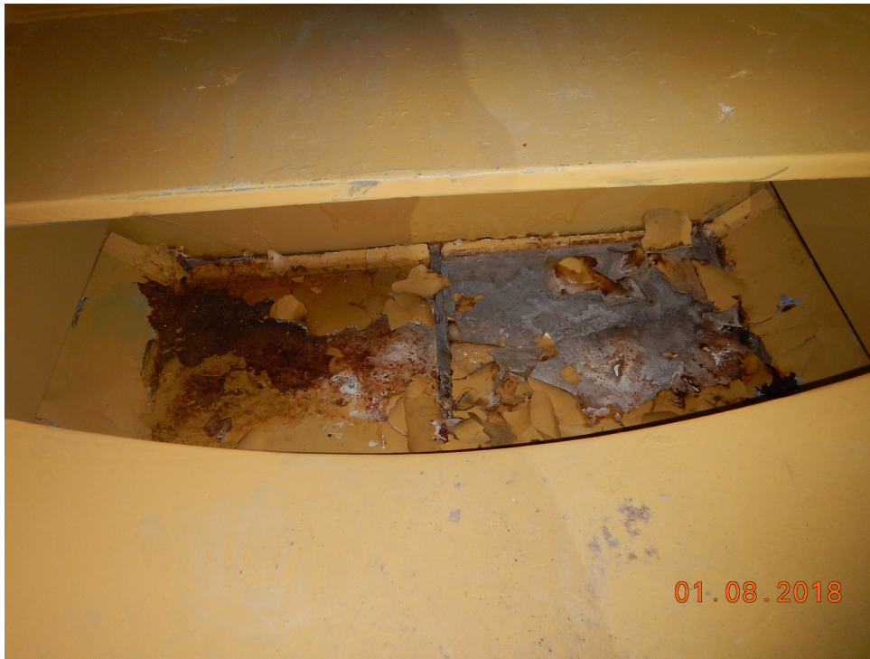
Figure 5.6: Corrosion trap on a Swedish bridge
