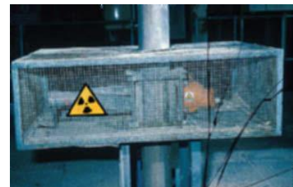
Figure 22: Installed density gauge mounted in housing (IAEA, 2003)
