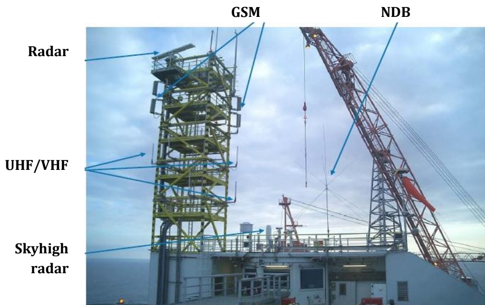
Figure 27: Different RF sources installed on an antenna tower. Adapted after: (Peikli, 2008 )
