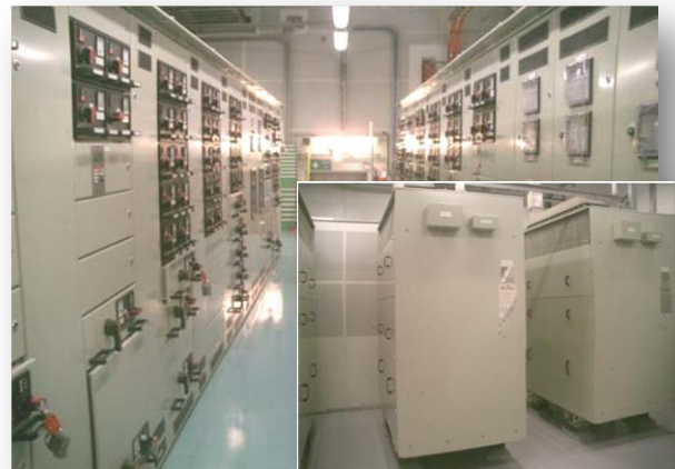
Figure 25: Low voltage switch gear room and LV transformer room (in the small picture) (Peikli, 2008 )
