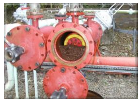
Figure 13: Pipeline pig at its arrival at the other end of a pipe (Pipeline Products & Services Association, 2014)
