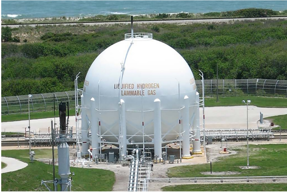
Figure 4.10: LH 2 storage sphere at KSC [44]
