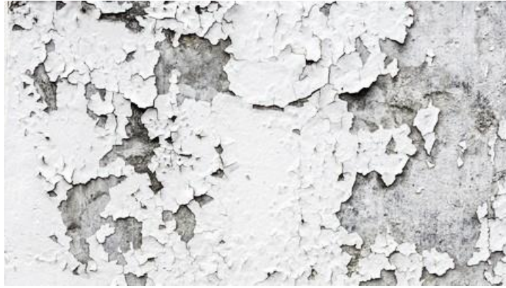
FIGURE 10: DELAMINATED CONCRETE SURFACE [12]
