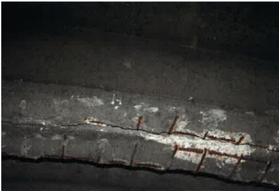
Figur 5-5: Eksponert armering betongelementer (Befaring 2005, u.d.)
